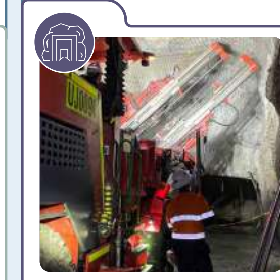
PYBAR awarded 4-year underground rehabilitation and development contract at Hillgrove Antimony-Gold Project, New South Wales, Australia
